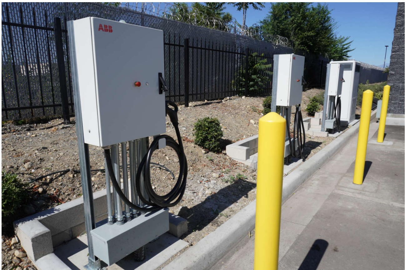
Figure 5. An example of outdoor charging infrastructure.
